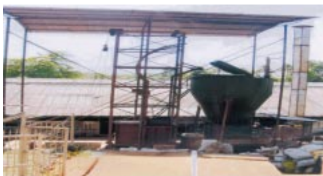
Biomass gasifier, 750,000 K Cals/hr installed at the 45 Tonnes/day TSR Factory of Pala Mktg. Co-op. Society Ltd at Pala.
